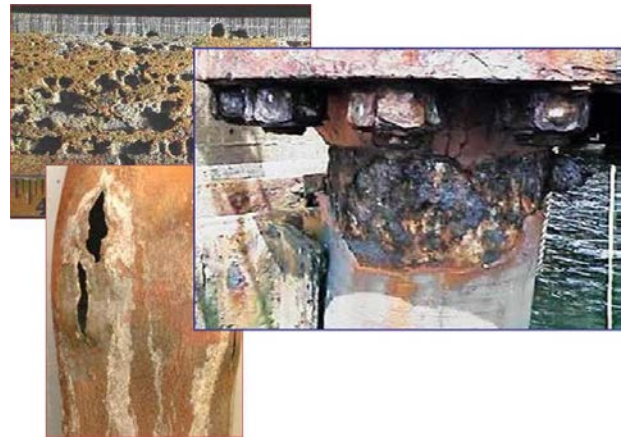
Figure 10. Viewing some deterioration mechanisms
